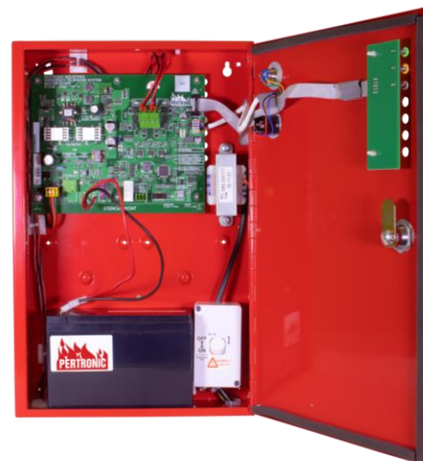
Pertronic Emergency Telephone System Master Controller, including master controller board, mains power switch, and battery
