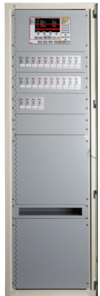
A 40U 14-loop F220 Fire Indicating Panel for a Queensland project. Below the keyboard & display, this large F220 features 24 fan control modules and a document tray. Pertronic fire alarm panels are available with white or grey front plates.
